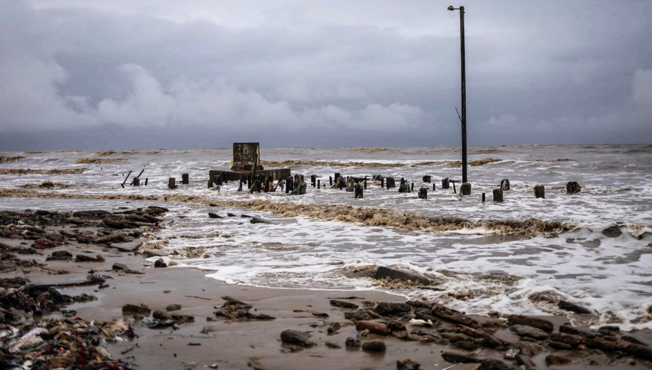
The skeleton of a power substation in Ayetoro lies broken and barnacled by the rising waters.
